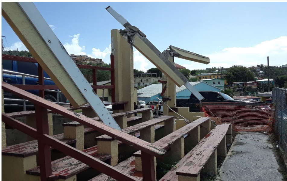
Pictured: Storm destruction on St. John near the school in Cruz Bay.
